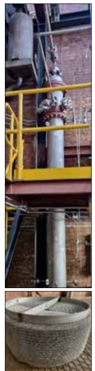
CO 2 capture pilot for industrial processes
