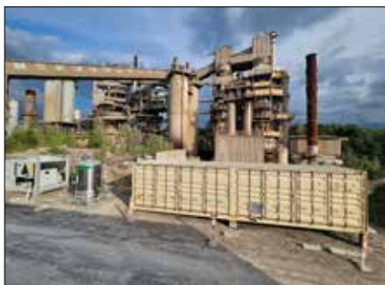
Fig 2 – Anti-sublimation cryogenic CO 2 -capture pilot (installed in lime production site)
